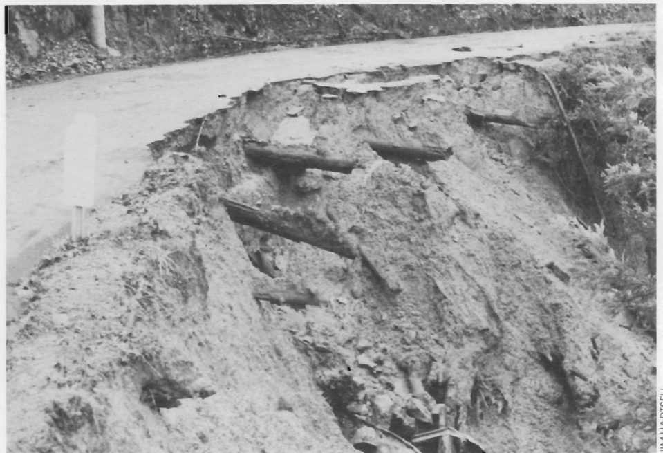
Picnic plans for HP Bay Area employees were in jeopardy when three sections of this road fell into the canyon in January. But the access road was repaired in time for the first picnic at the Little Basin recreation area.
